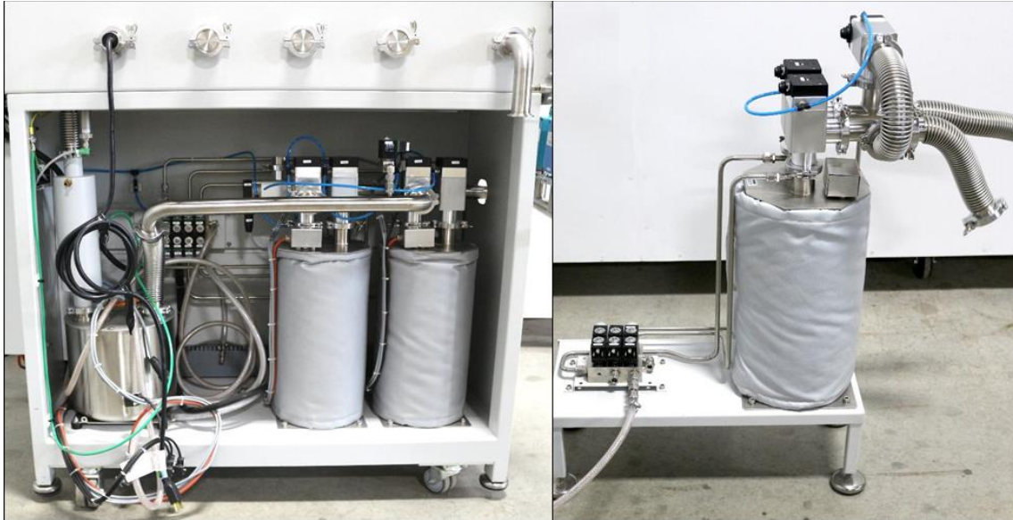
Figure 8: Left: Example of a purifier system with two separated canisters. These canisters can be duplicates, each containing a mixture of molecular sieve and copper catalyst OR the first canister contains the molecular sieve or the activated carbon and the second one contains the copper catalyst. Right: Example of a purifier system with only one canister containing a mix of molecular sieve and copper catalyst.
