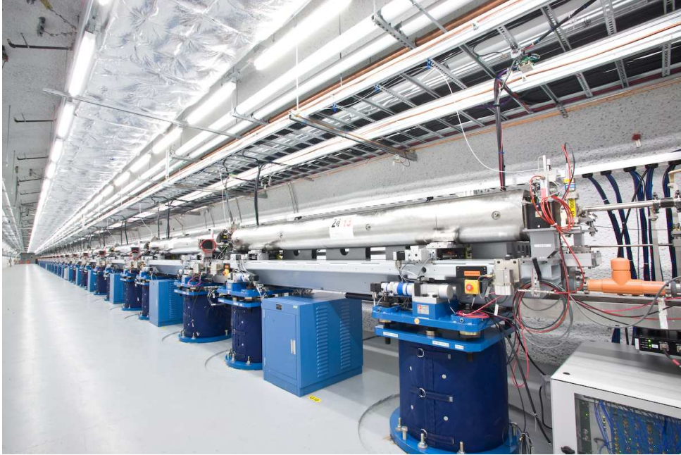
Figure 7: Photograph of the LCLS undulator hall. In the foreground, an undulator covered by a protective shield can be seen on its two pedestals [12].
