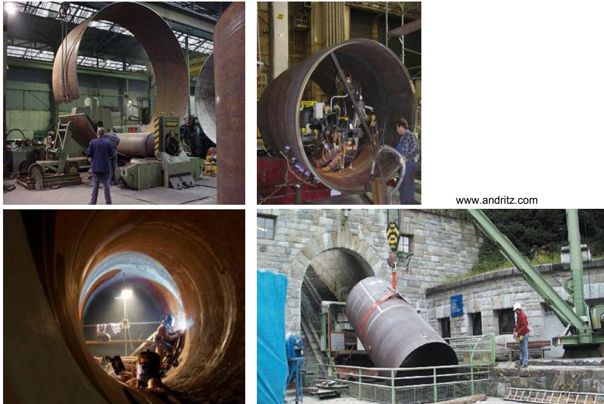
Figure 1: Fabrication et montage des blindages en acier / Manufacturing and erection of steel liners
