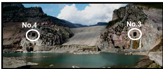
Figure 1 : View of the downstream face of the Koman dam with eroded dam toe and the outlet works
