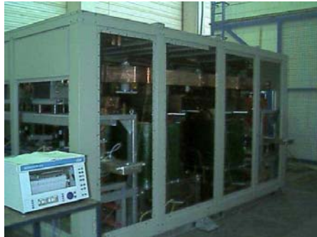
Power supply module (with transformers, interphase reactors, thyristor rectifier) during a test
