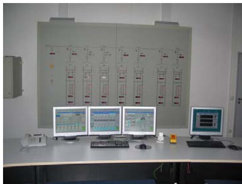
Control room of the power supplies
